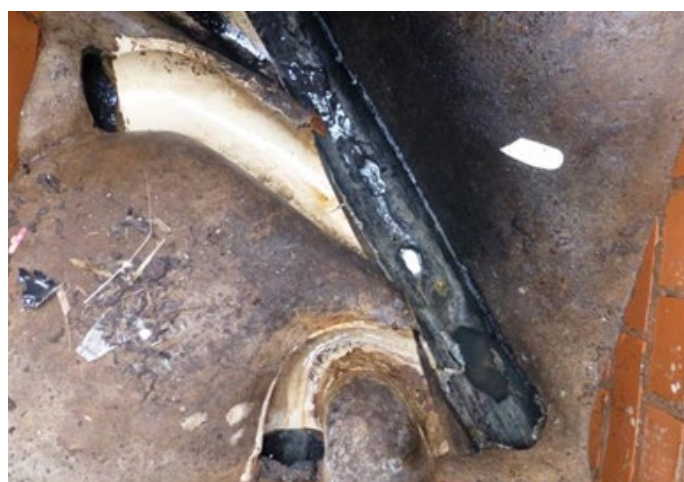
Figure One: In this inspection chamber, the main channel is formed by a pitched fibre pipe. This is unusual pitch fibre normally changes to salt glazed channels within the chamber.
