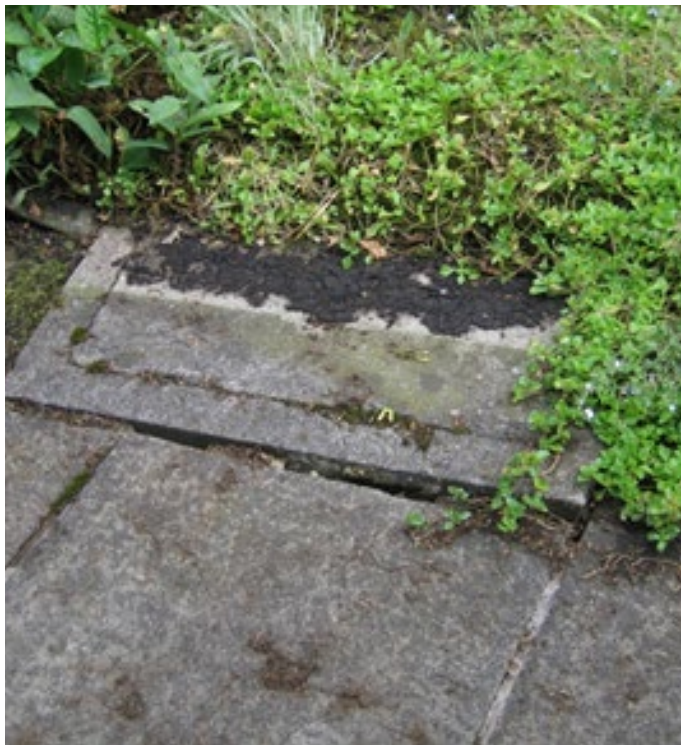
Figure two: This half-hidden inspection chamber has a tight fitting concrete cover. Not only would the cover be too heavy to lift but it looks to be stuck fast in its frame. You should record this in your site notes, take a photo and tell your client in the report.
