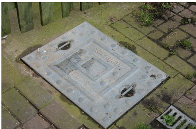
Figure three: Although this lightweight frame had a lot of debris between the cover and frame, we think you should take a little time to clear this so a full inspection can be carried out.
