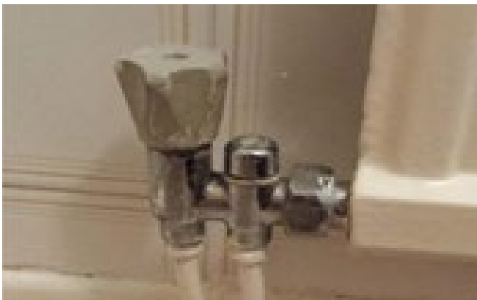
Figure 3 – Twin entry valves
