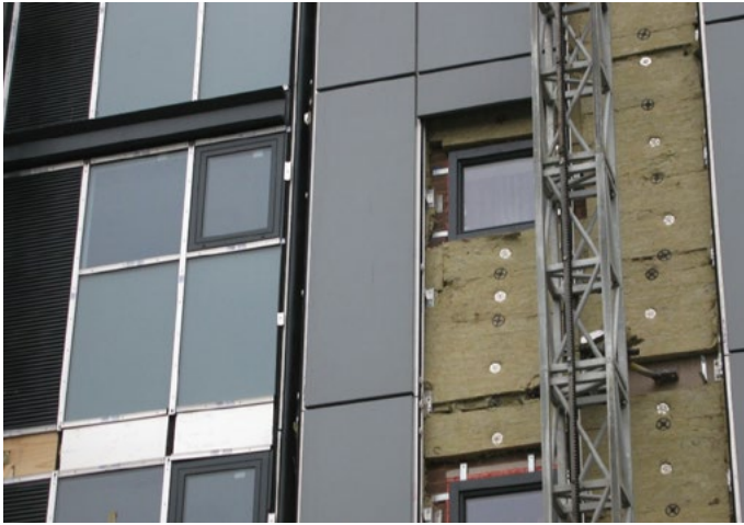
Figure 1: A rainscreen over-cladding system fixed to an existing 1950s block, approaching completion. The rainscreen is solid aluminium panels with mineral wool insulation. If installed properly, this would probably be considered low risk.
