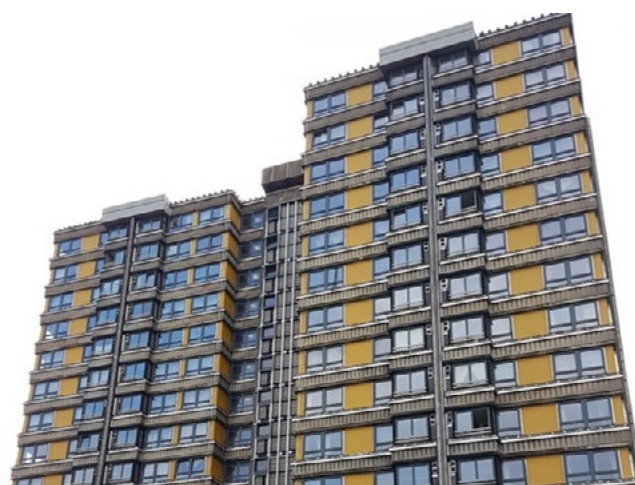
Figure 2: Local authority residential block with Category 3 ACM installed in 2009. It was removed, and replacement is still under discussion.
