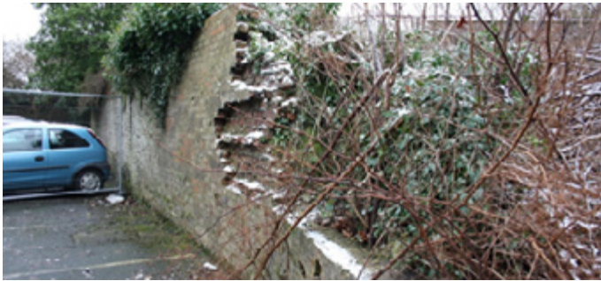
Figure 2: Japanese knotweed rhizome (root) growth causing the collapse of a section of wall in Stranraer (courtesy of Brian Taylor). © The Knotweed Company 2019
