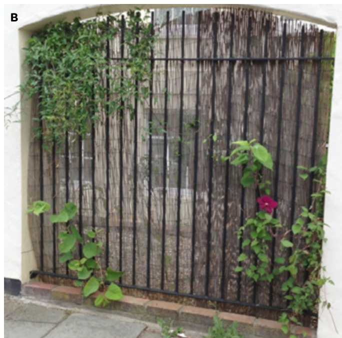
Figure 4: Japanese knotweed growth from unsealed gaps in laid concrete; (A) Southampton and (B) Bristol. © Daniel Jones 2019
