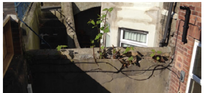
Figure 1: Japanese knotweed causing superficial damage to a wall in Cardiff. In this case, it was likely that contaminated soil was included in the mortar. © Daniel Jones 2019
