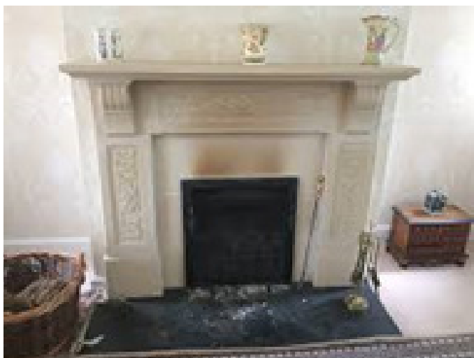
Figure 1 – signs of spillage on the fireplace mantle
