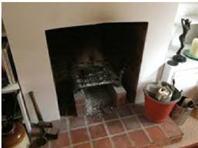
Figure 2 – signs of spillage above the open fireplace
