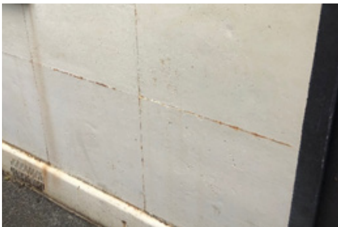
Figure 4 - View of the external painted wall panels, showing early stage corrosion to joints - this is why they are re-decorated regularly to prevent further, more serious deterioration
