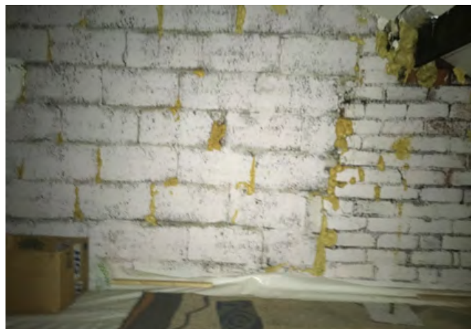
Figure 4 – expanding foam in all the cracks and in the top right of the image around the purlin.
