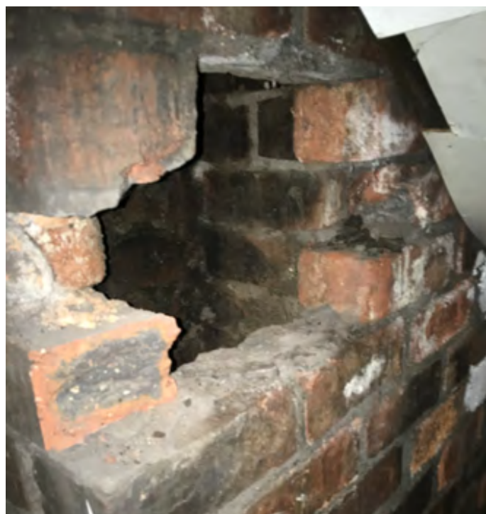
Figure 5 – hole in chimney (note the rough hole with no consideration for structural support of the chimney stack).
