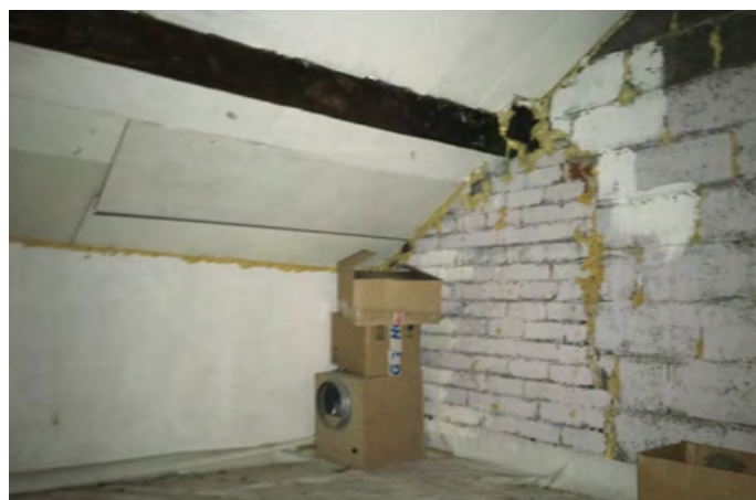
Figure 3 – plastic sheeting to the floor, roughly boarded over rafters and expanding foam to fill cracks.
