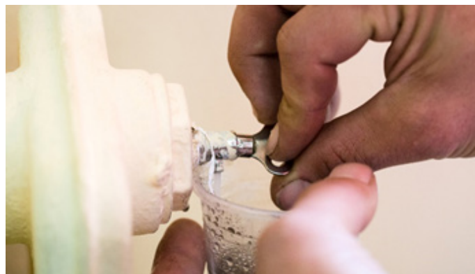
Figure 6 – bleeding a radiator
