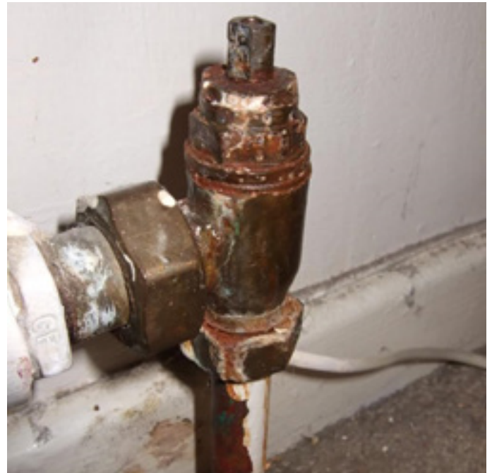
Figure 4 – example of scaly deposit on radiator valve
