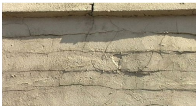
Figure 2: Cracked render above brickwork affected by sulphate attack
