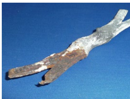
Figure 1: Rusting cavity wall tie
