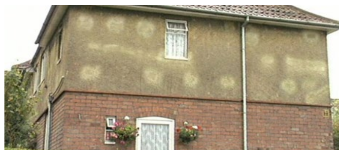
Figure 11: mismatched repointing, credit: www.designingbuildings.co.uk
