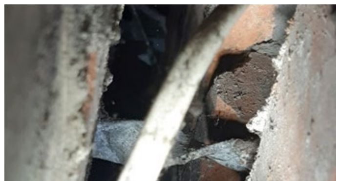
Figure 5: Wall tie with visible rusting
