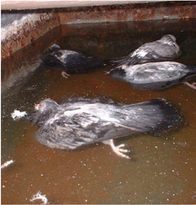
Figure 3: Contaminated water tank
