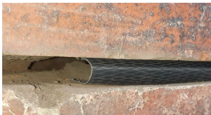
Figure 9: Plastic isolator hood
