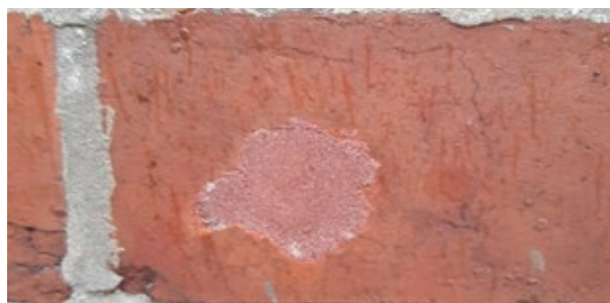
Figure 12: Drill hole evidence through brick
