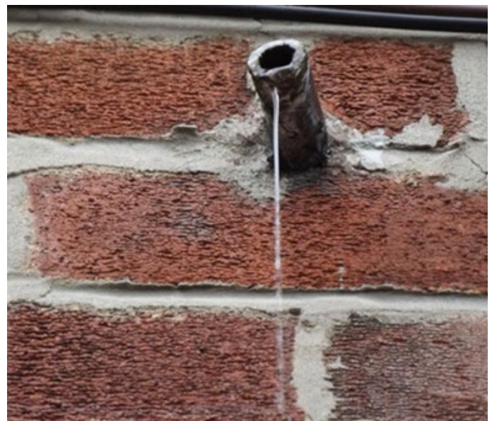
Figure 2: Dripping overflow pipe
