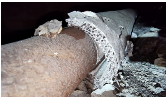
Figure 7: A close-up showing a cross section of this form of insulation. It is visually similar to cardboard, but the ‘corrugations’ are formed of paper containing high volumes of white asbestos.
