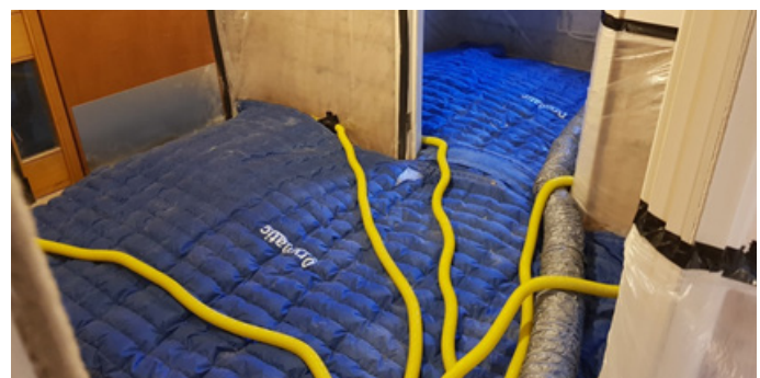
Figure 20: professional water removal following a flood
