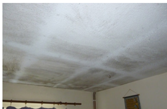
Figure 4 and 5: mould growth from moisture in cold spots. Photo credit: Robert Vaughan, Harlow Council
