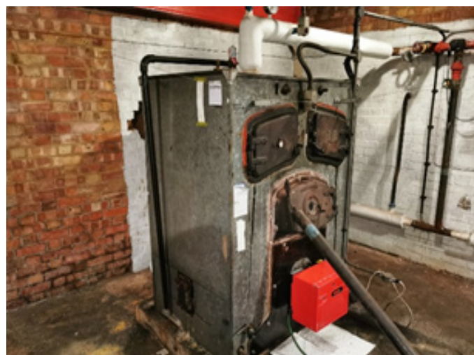
Figure 4: This Robin Hood cast iron sectional boiler dates back to the 1960s. It serviced a large warehouse before eventually being put out of commission. Beneath the galvanised steel casings are residues of more hard-set insulation, remnants of historic removal attempts.
