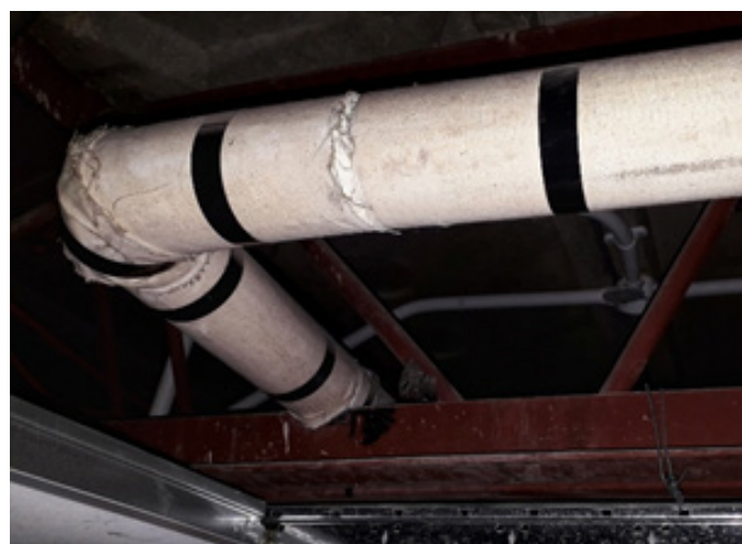
Figure 5: An example of asbestos magnesia sectional block insulation wrapped in a non-asbestos textile.
