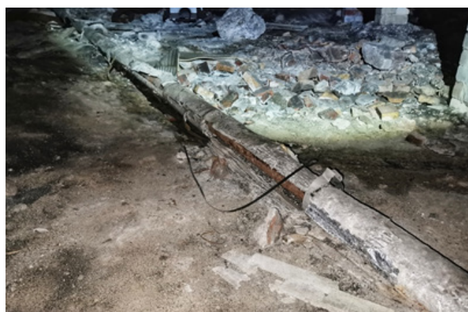
Figure 6: A long run of redundant pipe covered in highly damaged ‘air cell’ thermal insulation, found in the undercroft behind the boiler room in Figures 3 and 4.
