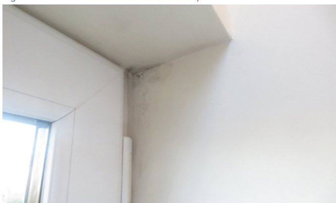
Figure 4: Black mould to corners of door reveals
