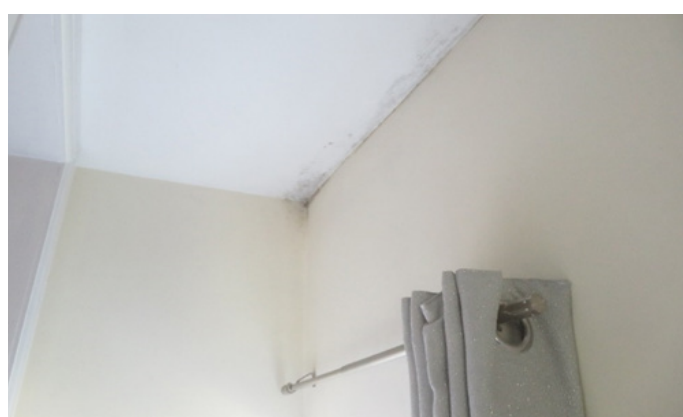
Figure 9: Black mould evident to corners of ceilings
