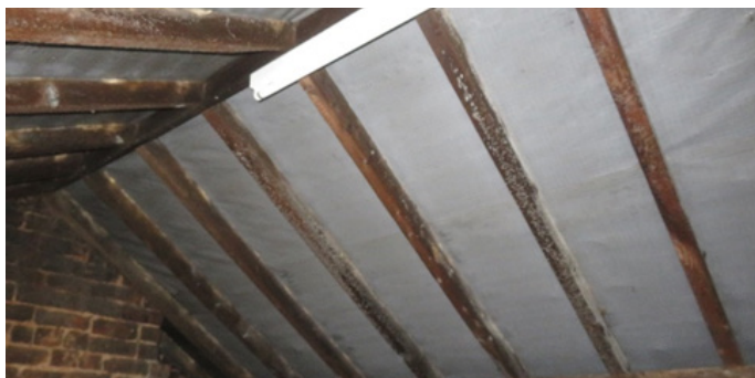
Figure 11: Mould growth evident to rafters
