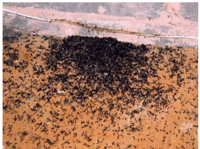
Figure 2: Close up of bat droppings on boarding
