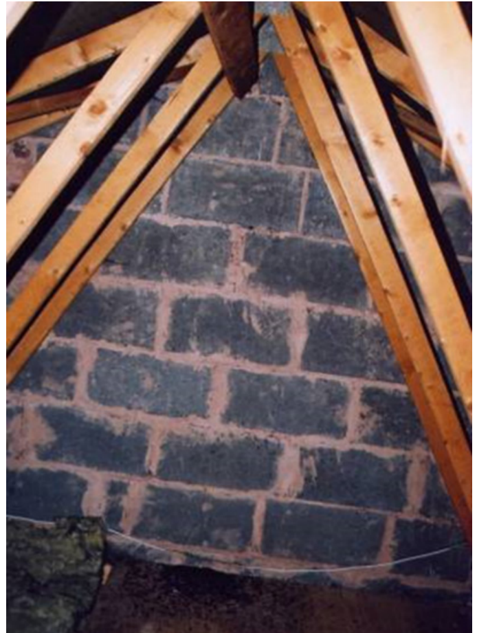
Figure 1: Gable end wall in context with bat droppings on boarding
