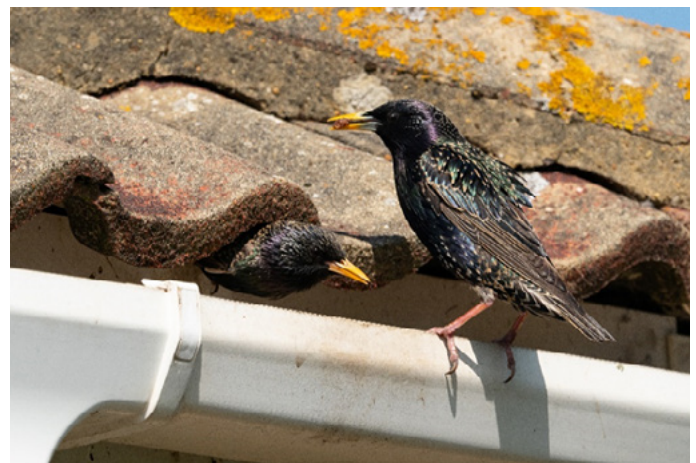
Figure 4: Starlings appearing from eaves of roof
