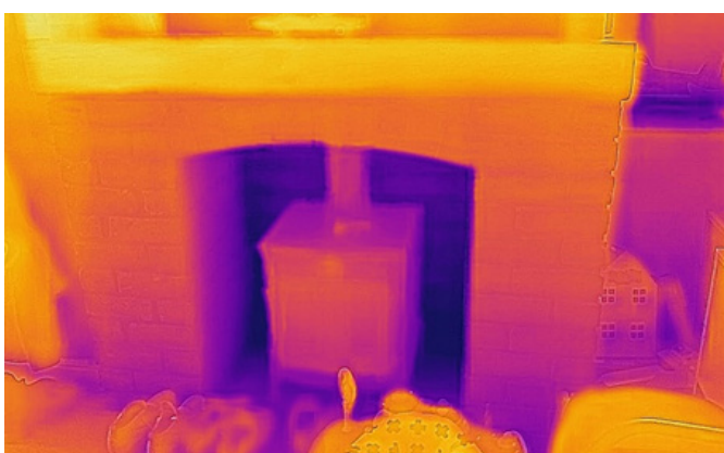
Figure 7: Cold bridging identified at rear of fireplace
