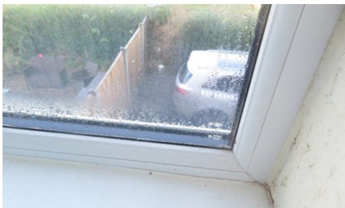
Figure 3: Condensation to windows internally
