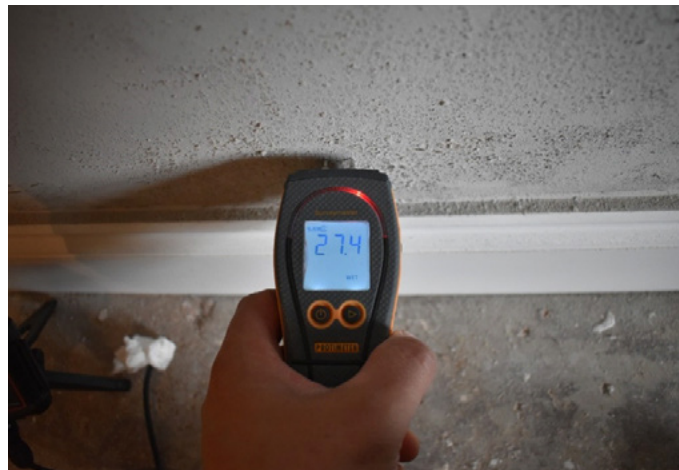
Figure 3: Electronic moisture meter revealing high readings when the spoiling plaster is tested
