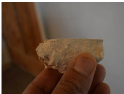
Figure 6: Inappropriate use of gypsum and cement renovating plasters during refurbishment
