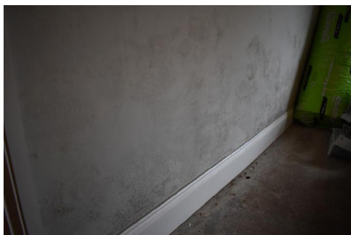
Figure 2: Distressed internal decorations which started to spoil shortly after the renovation was completed
