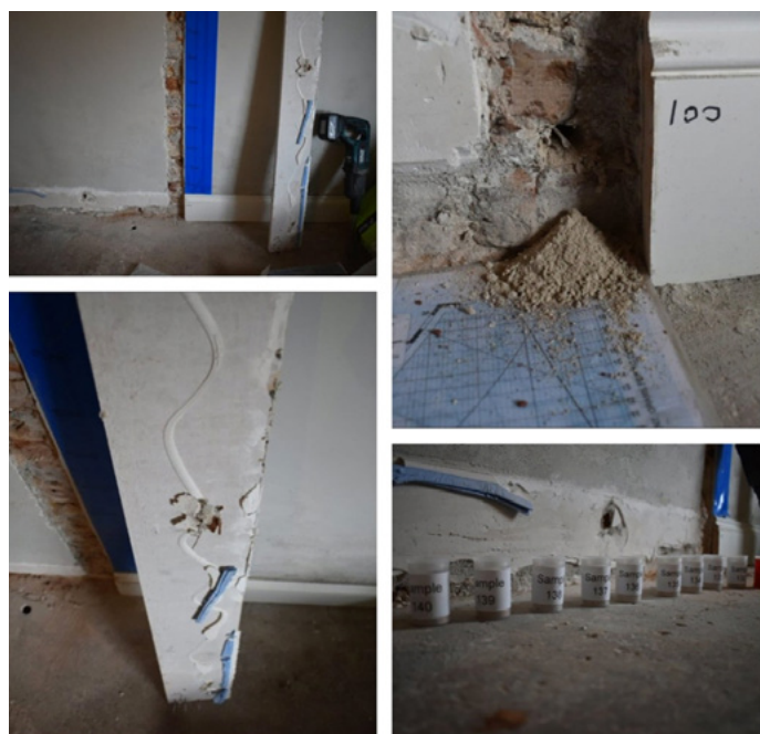
Figure 4: Samples extracted from the problematic walls for offsite moisture and salt analysis
