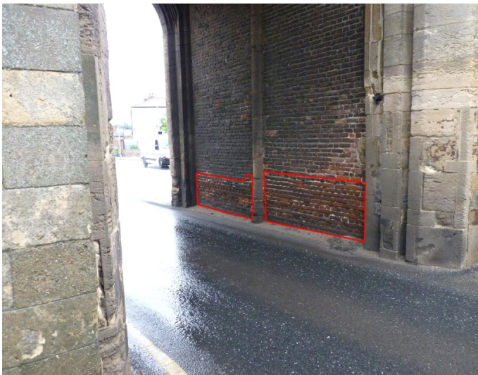
Figure 3: The South Gate, areas showing deterioration before repointing works
