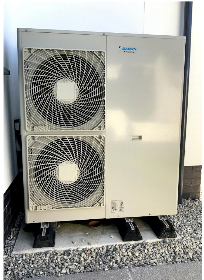
Figure 2: Air source heat pump unit
