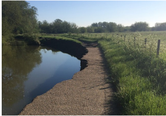
Figure 1: Visible damage to footpath adjacent to the River Great Ouse following flooding event.
